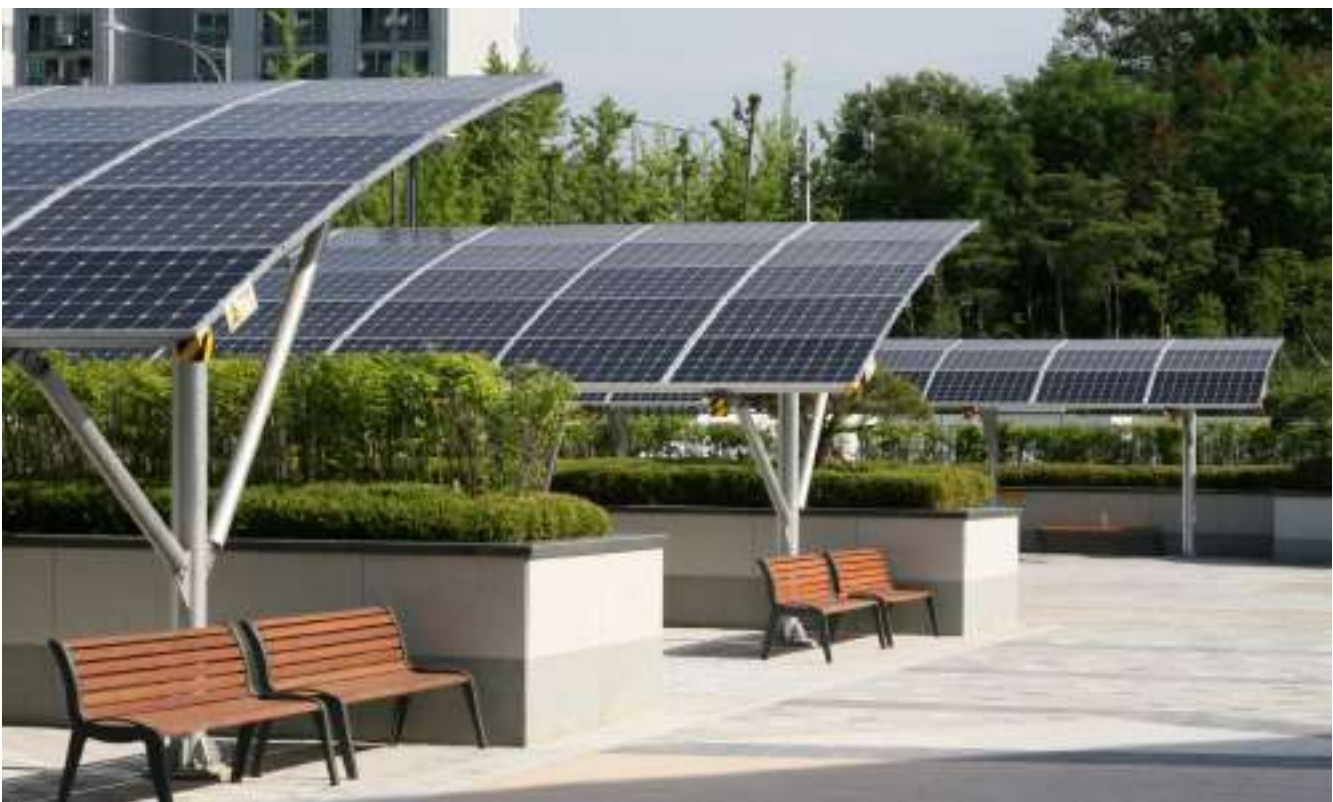
Solar Panela at a parking lot © KIM JIHYUN/Shutterstock
