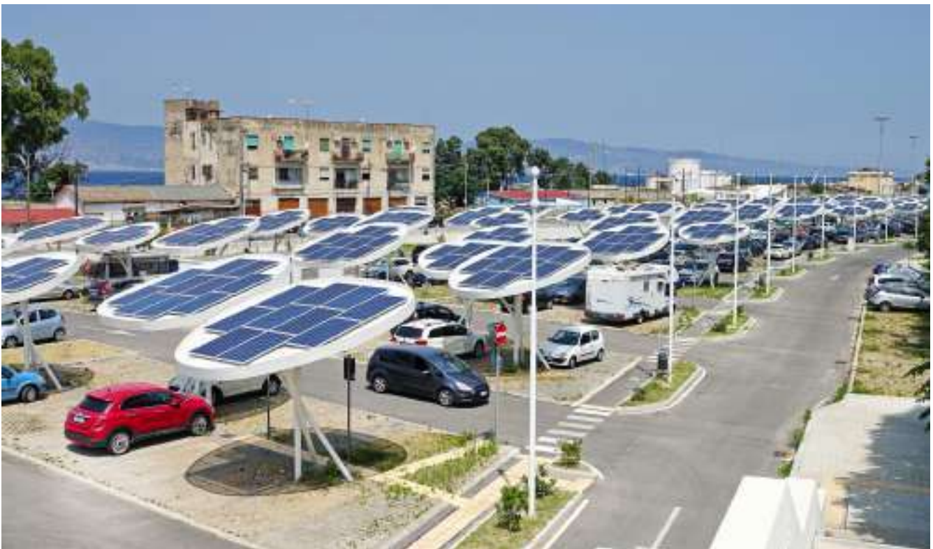
Solar panels in a car park. Companies are installing renewable energy sources to reduce their carbon footprint. Reggio Calabria, Italy
