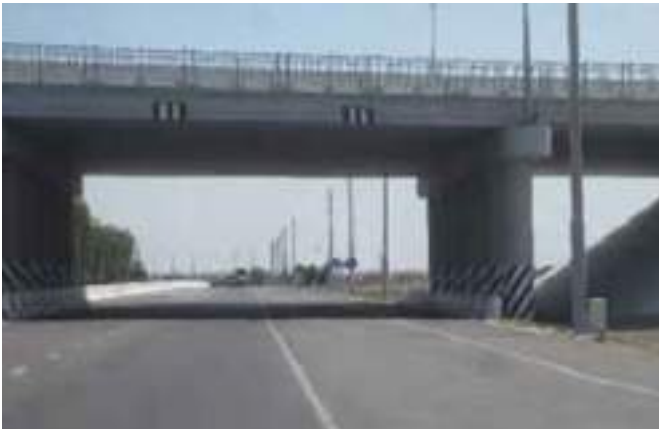
Figure 5.68: Unshielded overpass piers.
