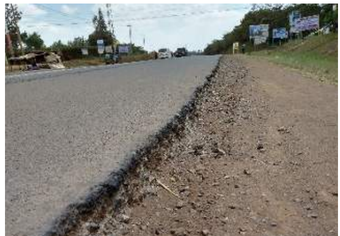
Figure 5.10: Pavement edge drop.
