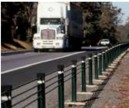
Figure 5.80: Flexible (wire-rope) barrier.
