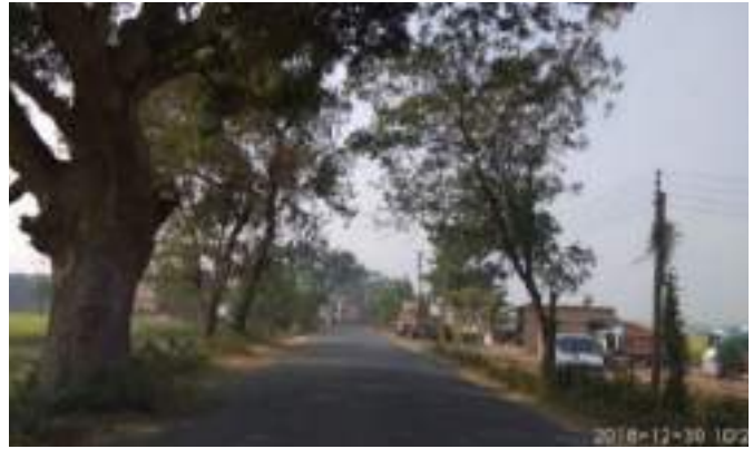
Figure 5.65: Trees (over 100 mm diameter) located too close to the carriageway.
