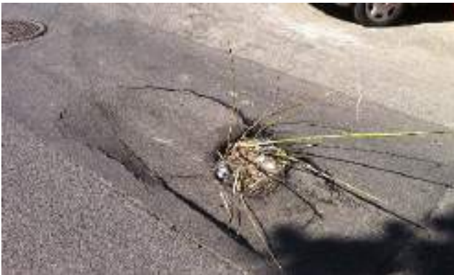
Figure 3.54: Poorly maintained road surface—Romania.
