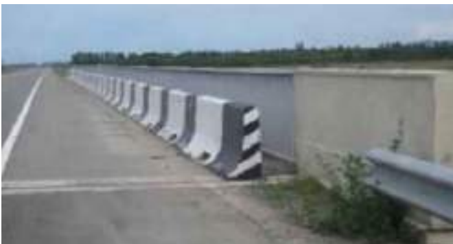
Figure 5.89: Unsafe gap between guardrail and concrete
