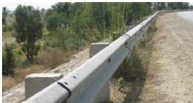
Figure 5.84: The rail units overlap in the wrong way.
