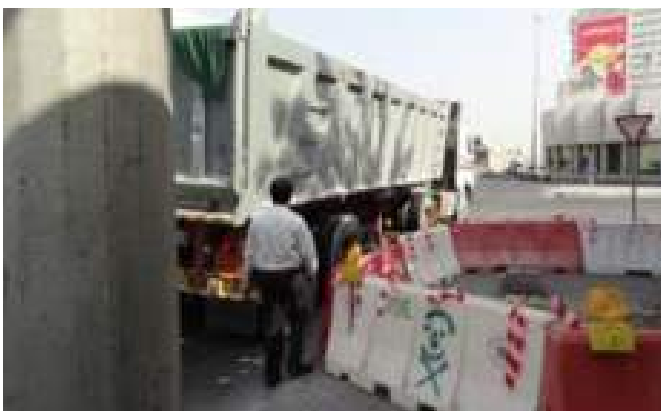
Figure 3.46: No provision for pedestrians—Qatar
