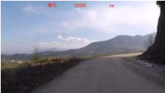
Figure 5.18: Insufficient delineation at curve.
