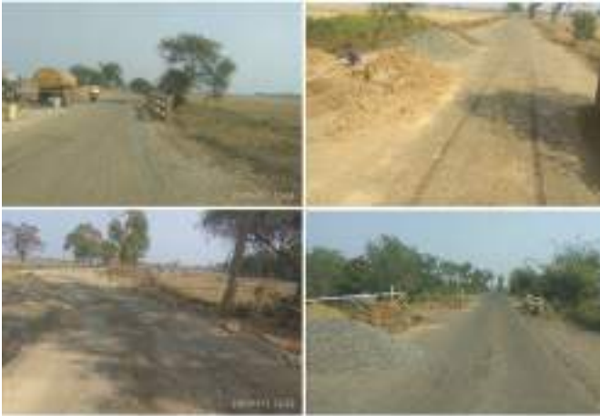
Figure 3.52: Unprotected work areas and materials—India
