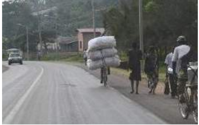
Figure 4.33: Cyclists on sealed shoulder with overlay to roadway causing level difference—Rwanda.
