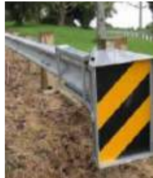
Figure 5.93: Flared energy absorbing terminal.
