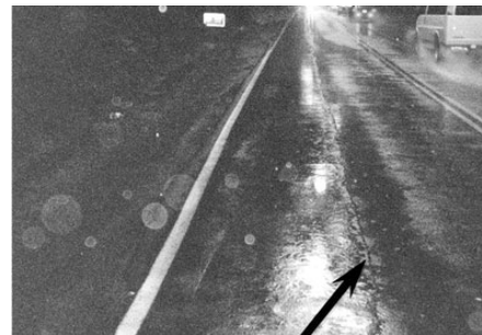
Figure 5.131: Edge of partial pavement overlay causing water to be retained on surface
