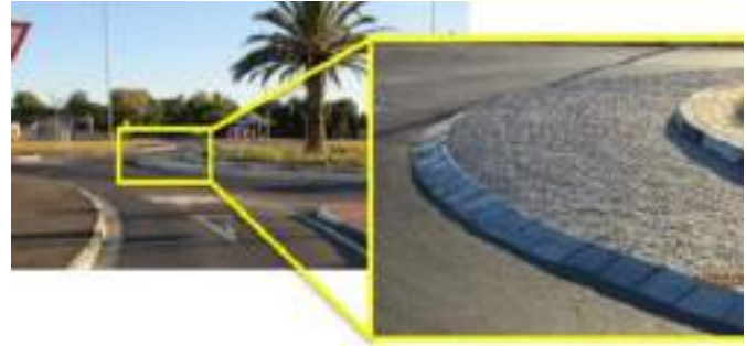
Figure 6.37: Truck apron with correct design for use by trucks only with a narrow circular carriage in South Africa.
