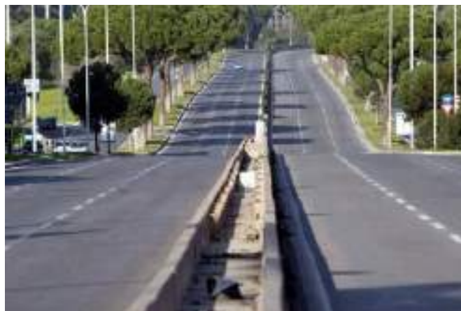
Figure 5.149: Hazardous vertical curbs on high-speed road.
