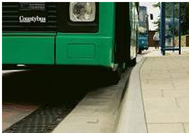
Figure 5.154: Bus-stop curb to ease passenger access.
