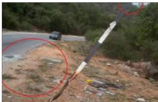
Figure 5.50: Broken signs without maintenance in India.
