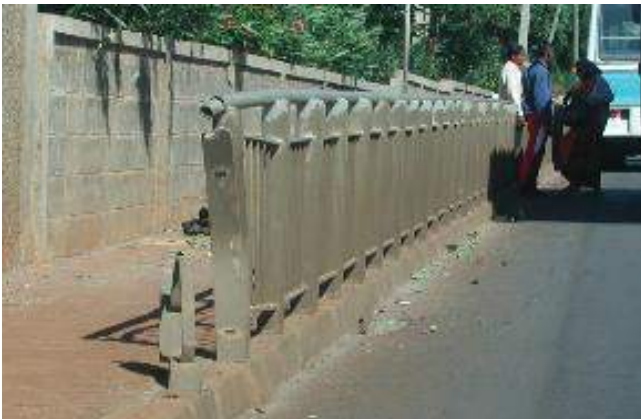
Figure 4.10: Poorly maintained pedestrian guardrail—Maintenance Inspection.
