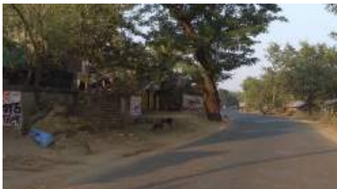
Figure 5.16: Tree located too close to the carriageway on inside of curve. It obstructs line of sight and is a safety hazard. It also has the potential to push road users toward or even across the centerline at a curve, making it very unsafe.
