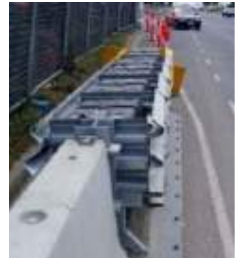
Figure 5.94: Safe crash cushion at the end of rigid barrier at a construction site.
