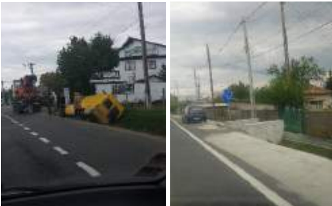
Figure 5.66: Uncovered drain and unsafe culvert—Romania.
