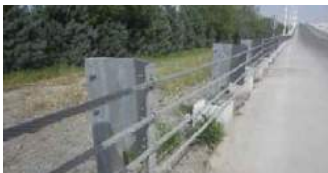
Figure 5.83: Flexible barriers with too large posts.
