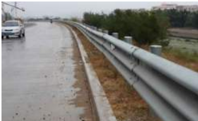
Figure 5.150: Example of dangerous curb-barrier combination with the steel barrier just behind the curb.
